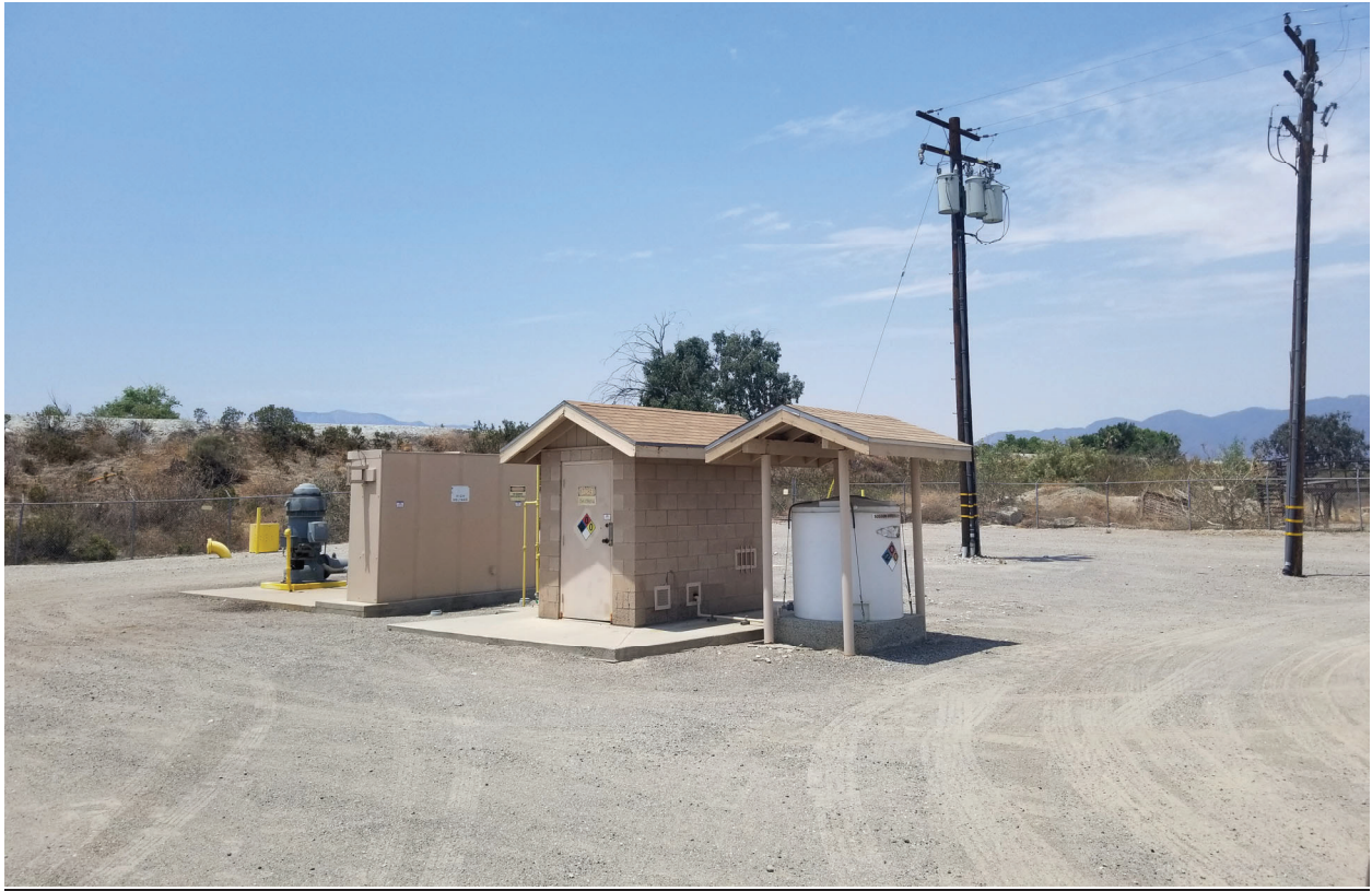
Address: 2015 W 9th St., San Bernardino, CA 92411 Pump Station 3A-1
