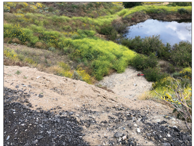
(Above) Looking north at Alder at failed road area (Below) Looking east downhill on Alder at failed road area
