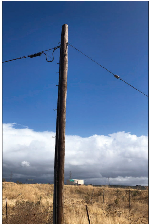
Existing Above Ground Cable to Underground at Freeway
