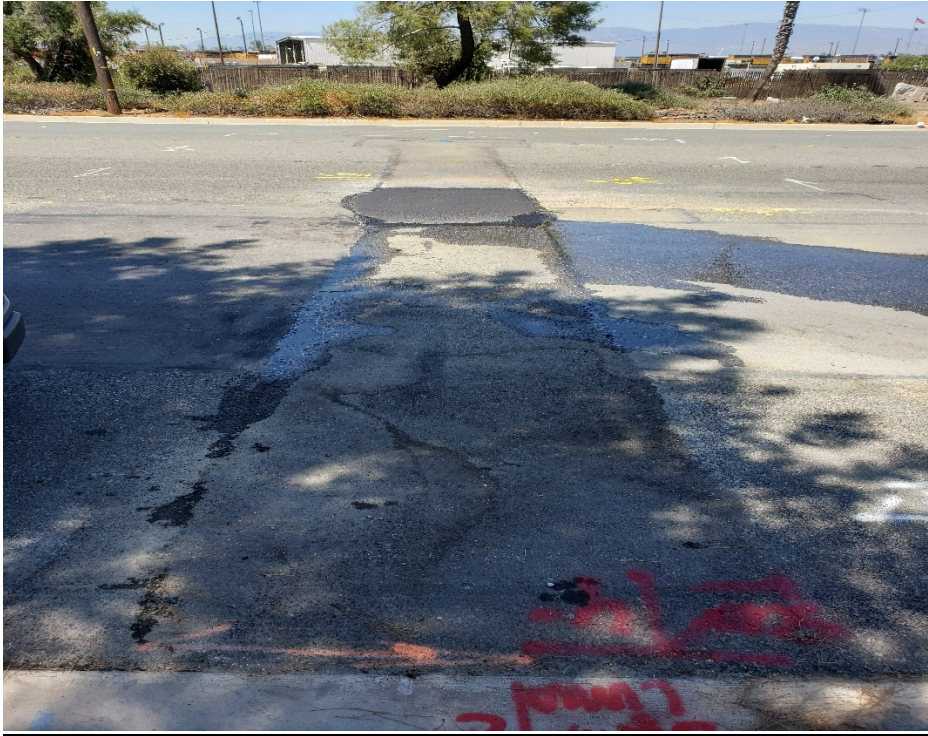
Photo of Leak
