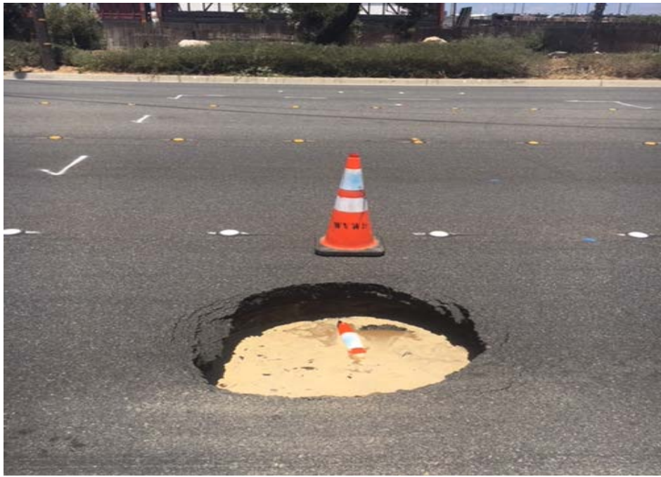
Sinkhole Formed Back in 2018
