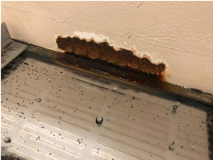
Example of the need for re-coating of tank interior. Near center flume of filter.
